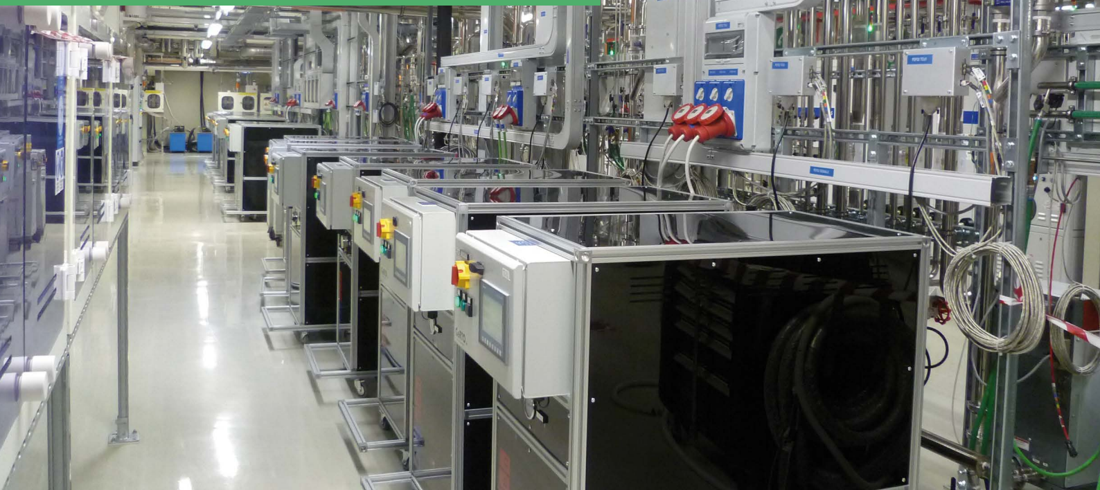
Thermal processing units, ST Catania, Italy
