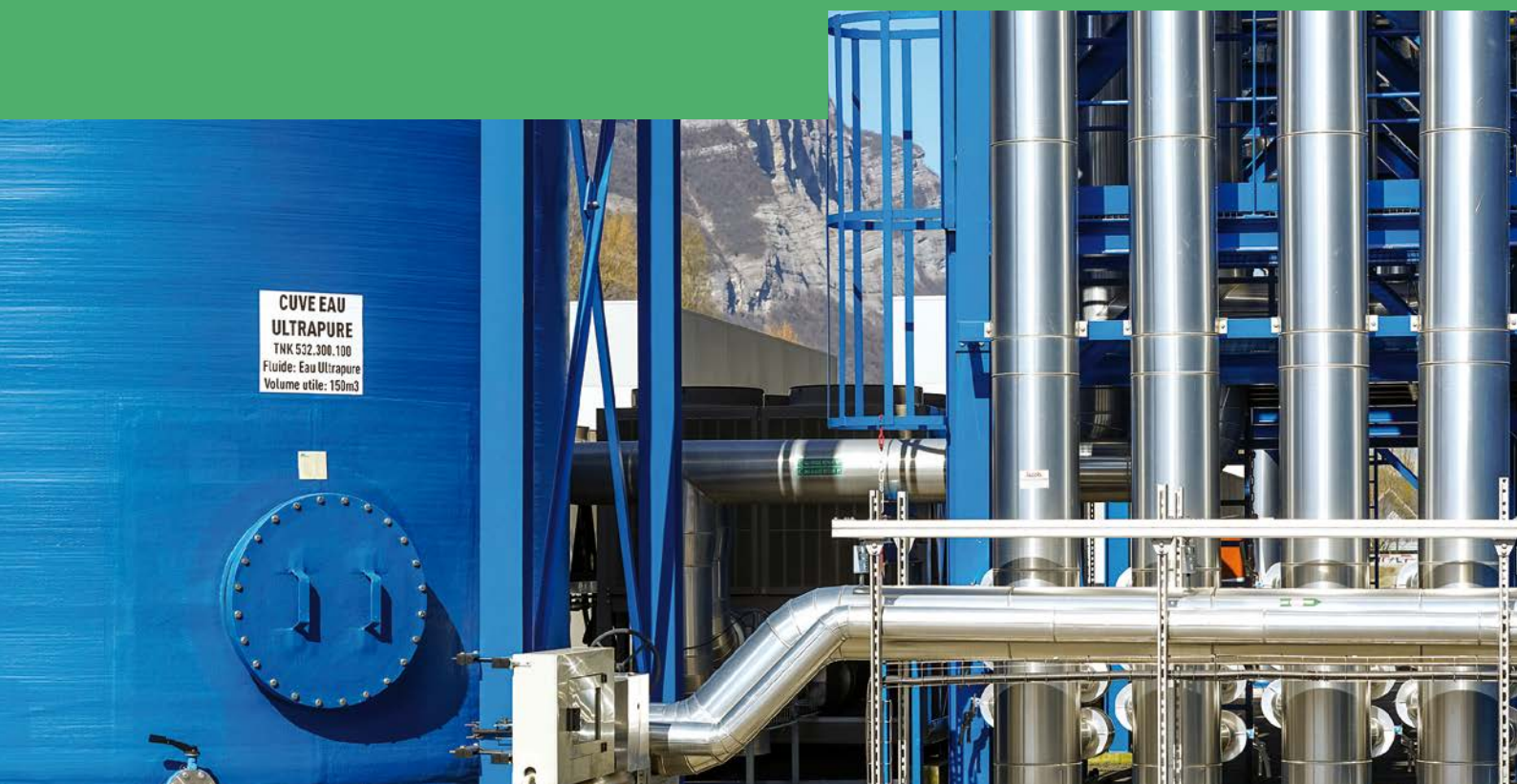
Ultra-pure water, ST Crolles, France
